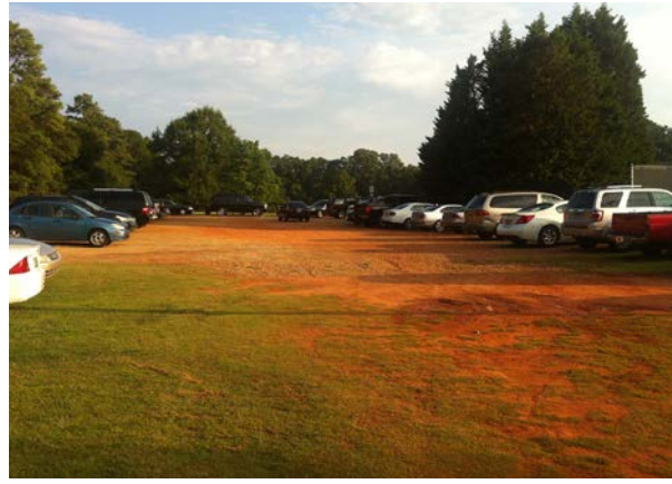
Figure A.6: Overflow parking erosion Daily use of overflow parking contributes to erosion.
