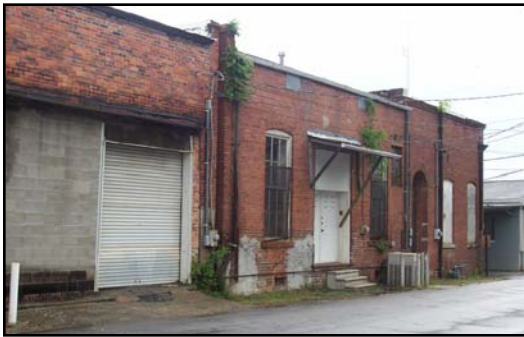
Boarded windows send a negative message to the visitor.
