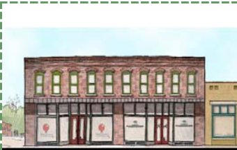
Very good example of a historic structure, only needs a more compatible awning.
