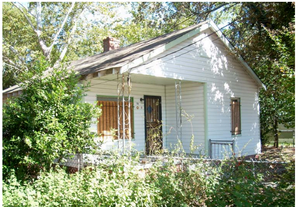
Photo 3: By contrast, bare, ill-fitting plywood does not protect the openings and makes the house – and the entire neighborhood – look abandoned, unfriendly and unsafe.
