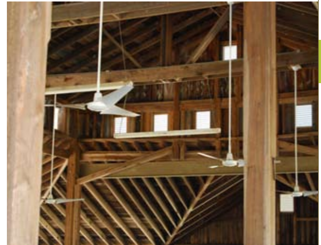
Exposed beams and timber-framing of the Methodist Campground site are good design elements to be incorporated into a new building aesthetic on the Research Forest site.
