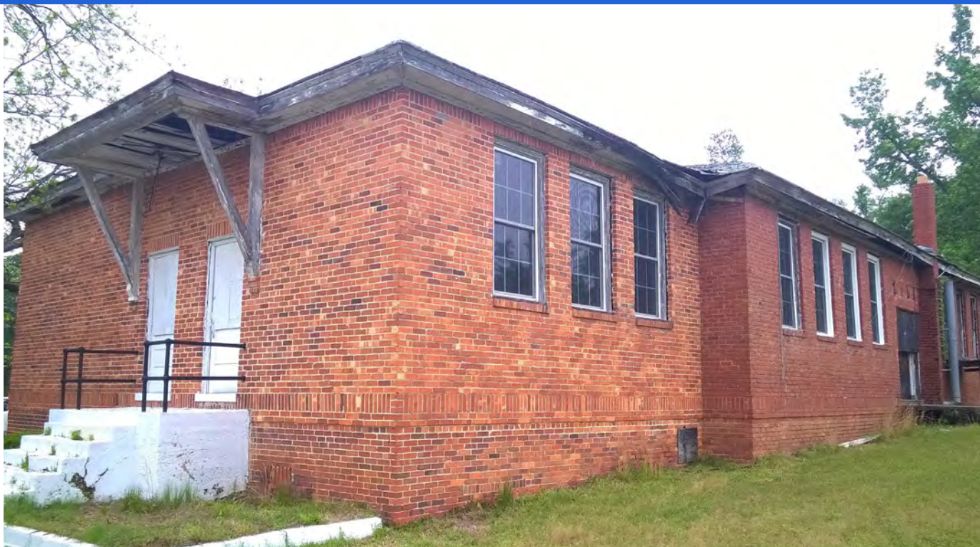
Roof damage is allowing water to penetrate the interior and deteriorate the soffits.
