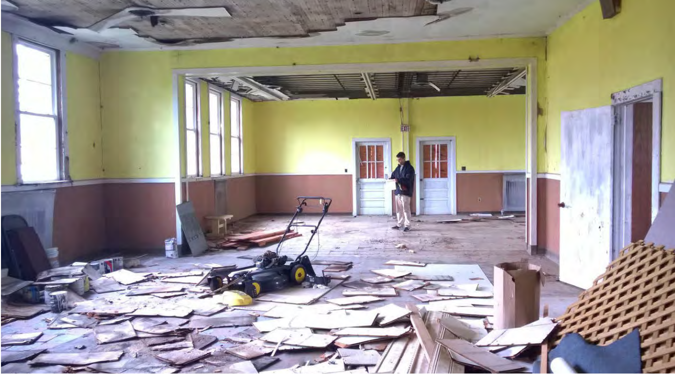
Existing condition of the Dining Hall. Roof is damaged and interior is filled with rubble.
