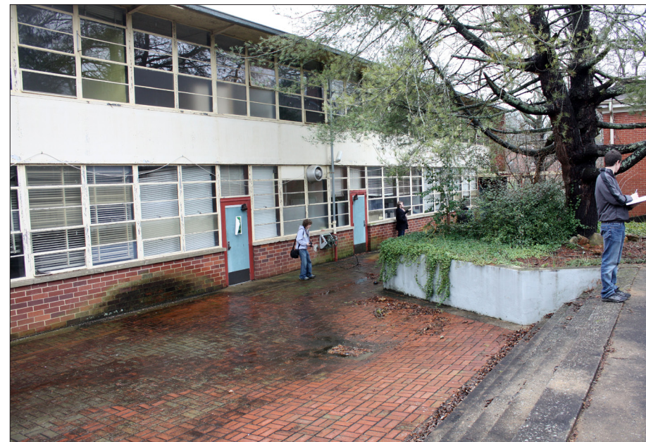
Current condition of courtyard. Simple maintenance and up-keep -- such as pressure-washing the brick patio to avoid slips -- would greatly improve the usability of the space.
