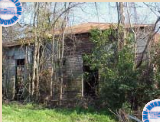
A structural assessment and feasibility study should be conducted for the depot.
