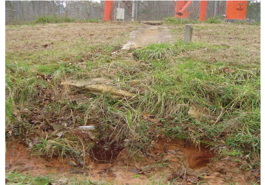
Erosion from pipe draining water tower
