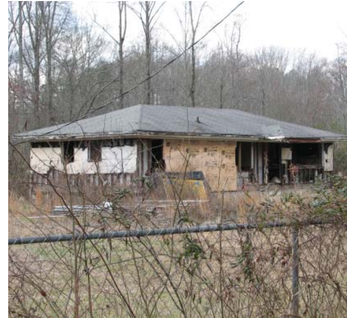
Dilapidated Housing or abandoned properties that remain unmaintained
