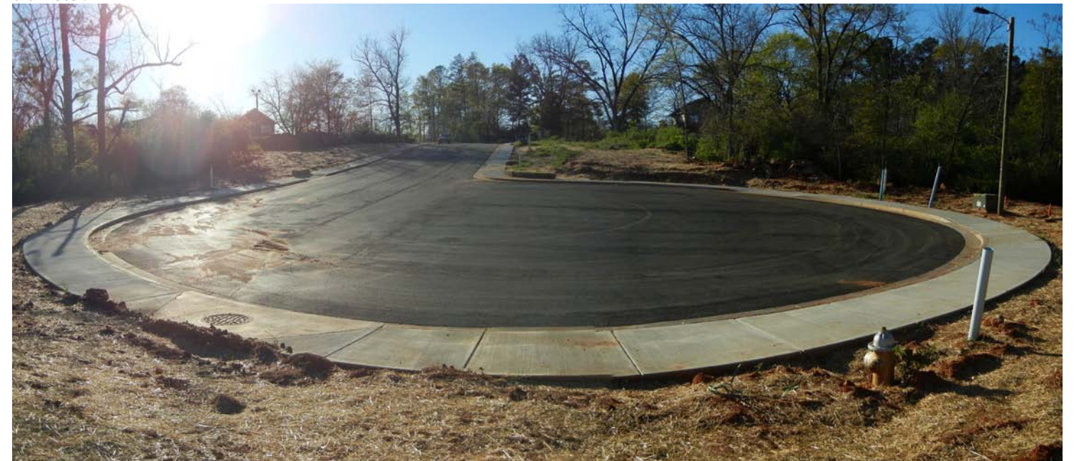
Figure 84 - Panoramic view of Cannon Drive cul-de-sac taken from the stormwater detention area looking towards Bray Street.
