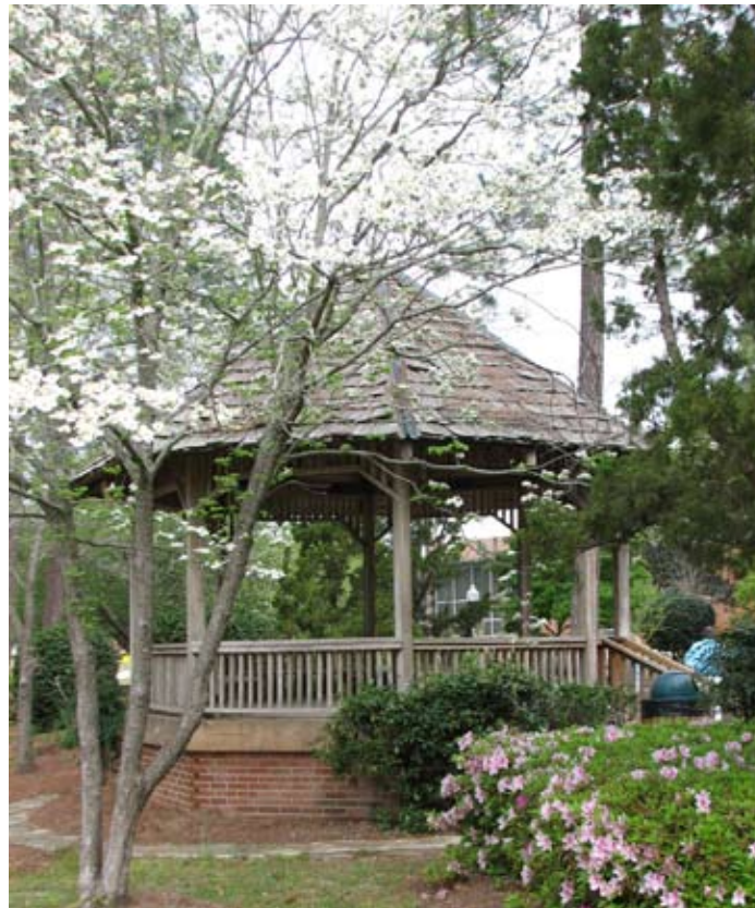
The wooden gazebo is being slowly demolished by carpenter bees and presents an unified appearance that detracts from the graceful and beautiful chapel, it removal would result in a more successful public space.
