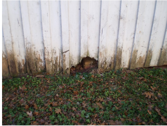
Termite damage on southeast corner, exposing brick pier
