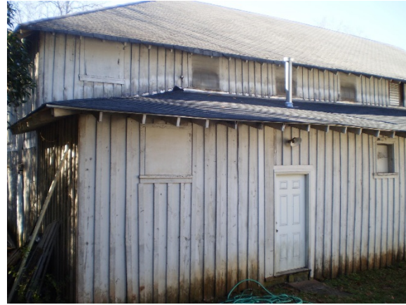
Note moss growing beneath the door
