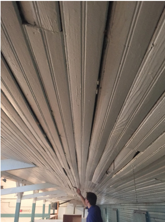
Damaged beadboard of southwest side over bleachers
