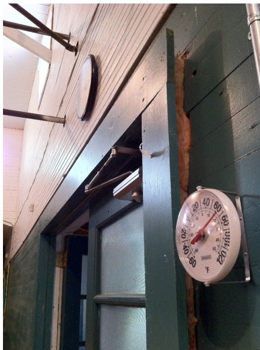
Interior of front gym wall, wall pulling away from door frame porch (exposed fiberglass insulation visible)
