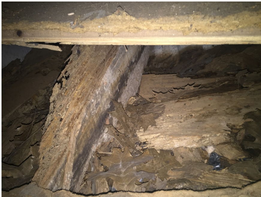
Floor of Home Team locker room, collapsed due to moisture and insect damage
