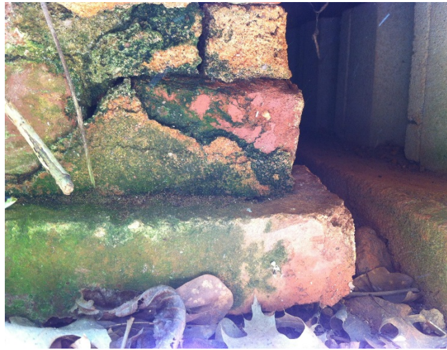
Brick pier at rear of building, overgrown with moss
