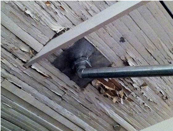
South corner heating exhaust damage
