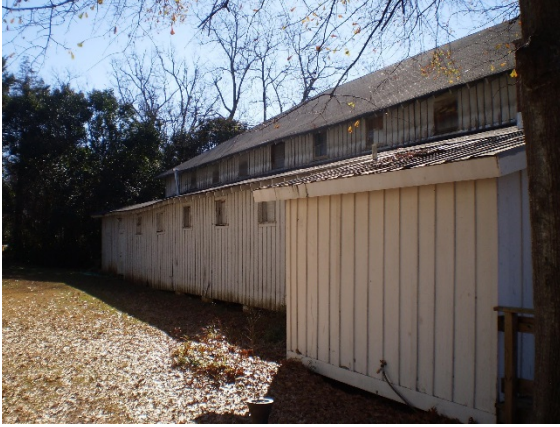
The southeast corner at rear with visible dip as it sinks
