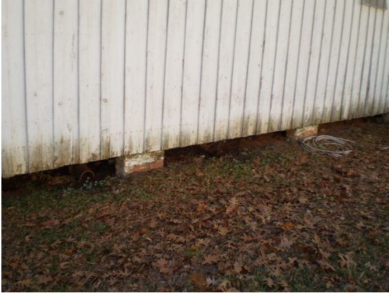
Overlapping wood siding with backsplash damage
