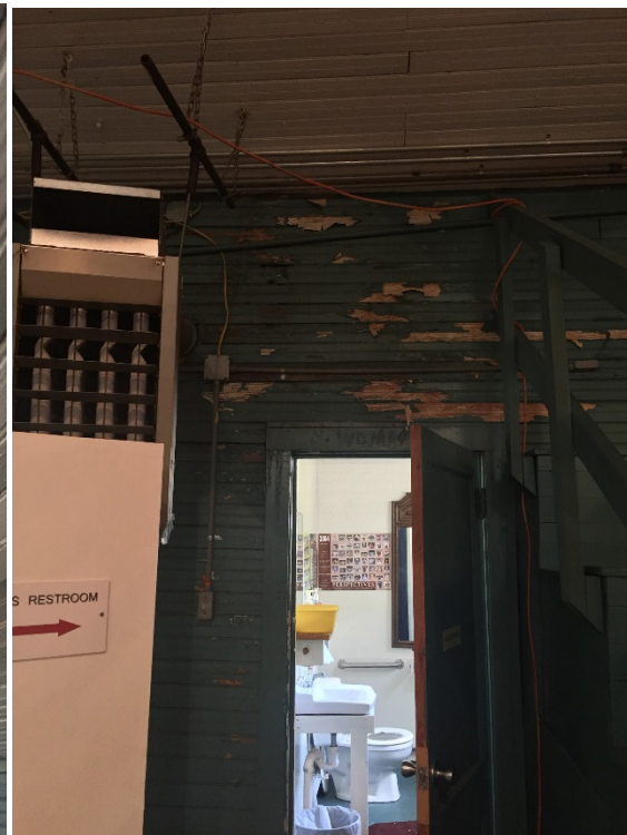
North corner bathroom additions with water damage
