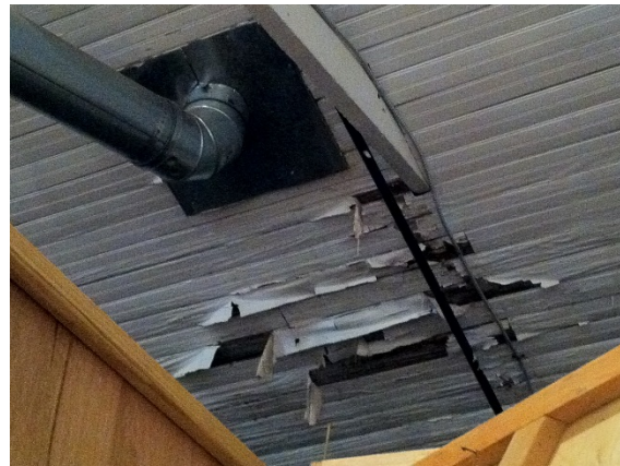
East corner heating exhaust damage
