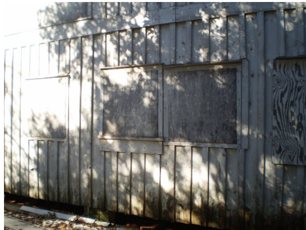
Moss grows on one of the brick piers, water damage along bottom edge
