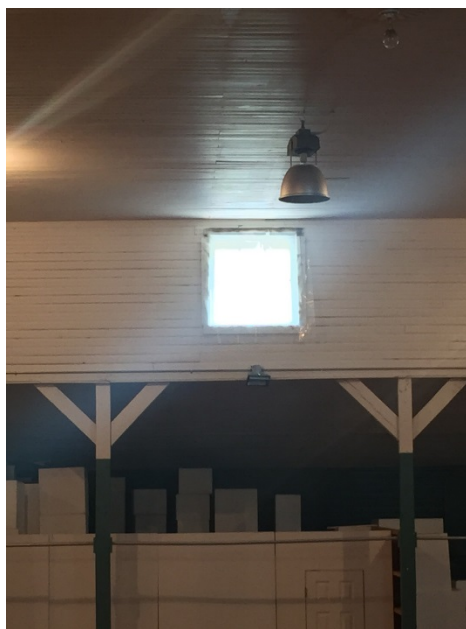
SW clerestory window, covered with plastic sheeting
