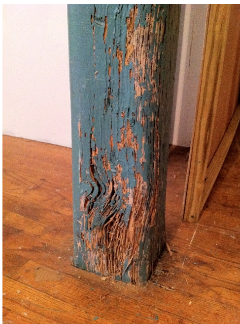
Supporting post in east corner of gym interior, termite damage
