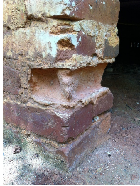
Moisture damaged, compromised brick
