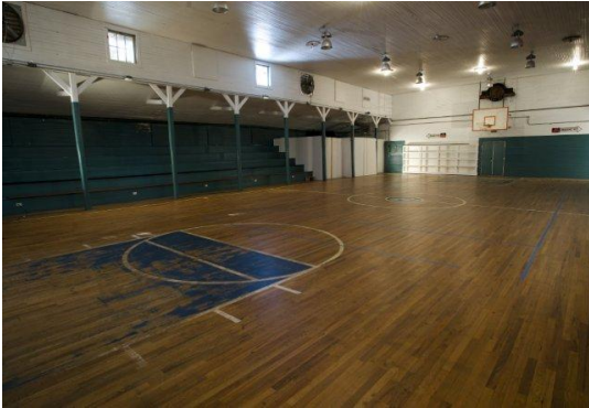
Interior view from W corner, looking at damaged SE corner
