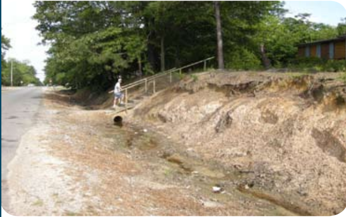
This is the most severe erosion found in the neighborhood.
