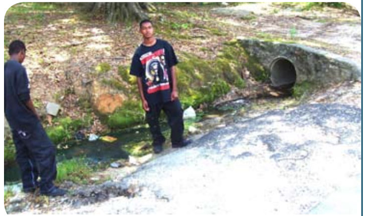
Trash and standing water are issues throughout the ditch systems.
