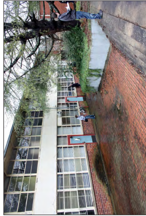
Current condition of courtyard. Simple maintenance and up-keep -- such as pressure-washing the brick patio to avoid slips -- would greatly improve the usability of the space.
